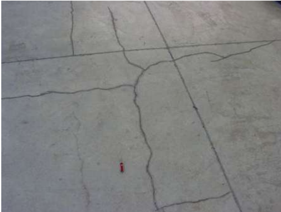
Fig2: Cracks developed due to expansion of concrete.
