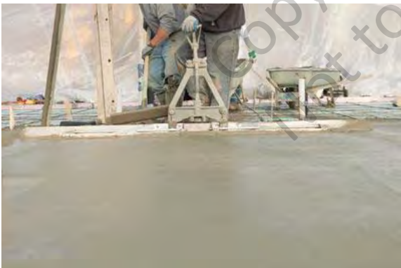
How to solve curling, cracking, scaling and more concrete problems
