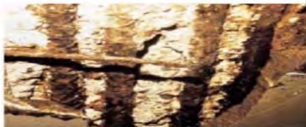
The damage to this concrete parking structure resulted from chloride- induced corrosion of steel reinforcement
