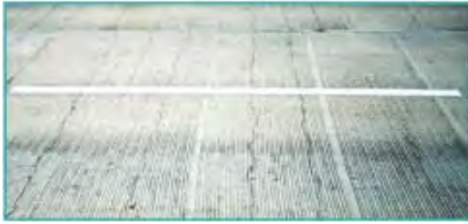
Shrinkage cracks, such as shown on this bridge deck, can be reduced with the use of good concreting practices and shrinkage reducing admixtures
