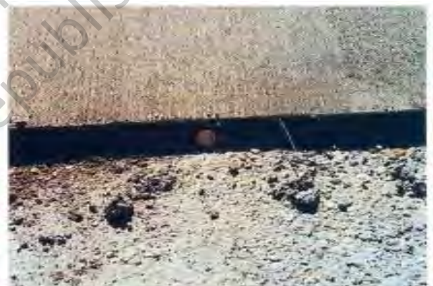
Plasticized, flowing concrete is easily placed in thin sections such as this bonded overlay that is not much thicker than 1 1/2 diameters of a quarter.
