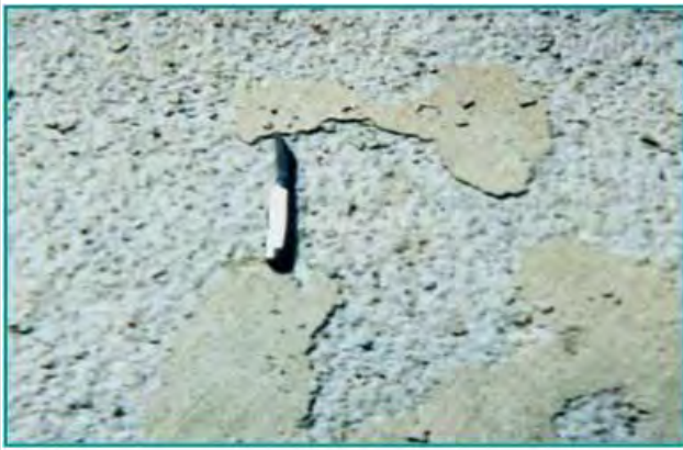
Scaled concrete surface resulting from lack of air entrainment, use of deicers, and poor finishing and curing practices
