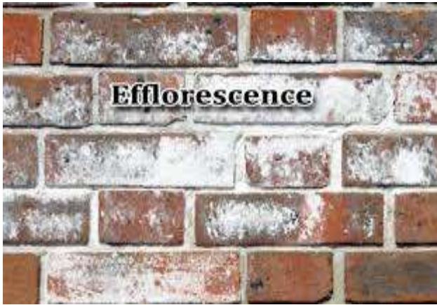
EFFLORESCENCE OF BRICK WORK
